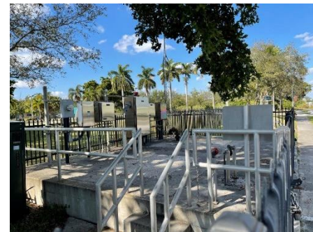
Lift Station N-7 located at 2402 Green St.
